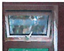
Keep windows open to let water vapour escape.
