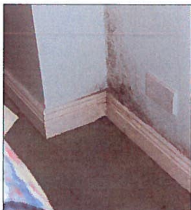
Mould growth in bedroom due to condensation.
