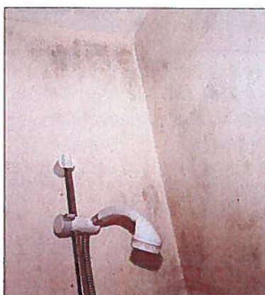
Mould growth in bathroom due to condensation.
