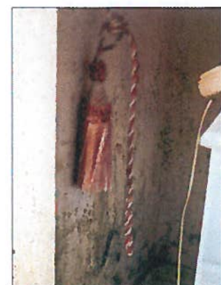
Mould growth due to condensation in corner of room.
