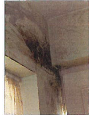
Mould growth due to condensation in hall.
