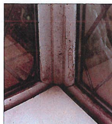
Mould growth on window frame due to condensation.
