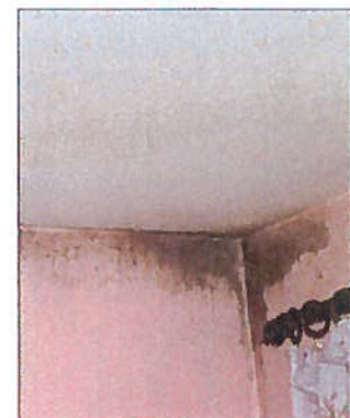
Mould growth due to condensation in corner of room.
